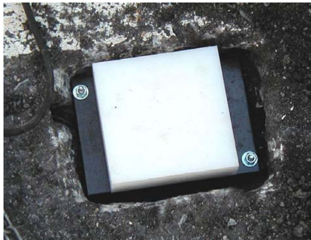
Figure 6: In-Road Antenna mounted with wedge anchor bolts
